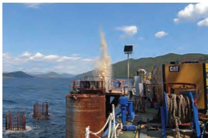
The attempt to remove the damaged part of the pile of the S12 pier foundation with explosives failed.
